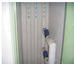
Wireless water meters installed on tube-wells
