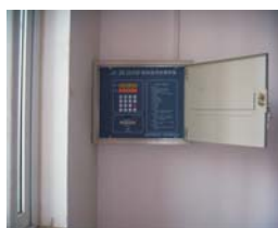
Wireless systems installed in the stairwell
